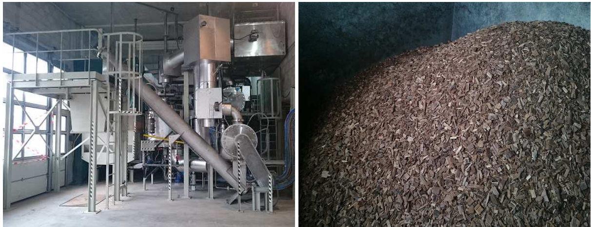
TORPLANT pilot plant unit in Orbe (CH) - capacity 100 kg/h
